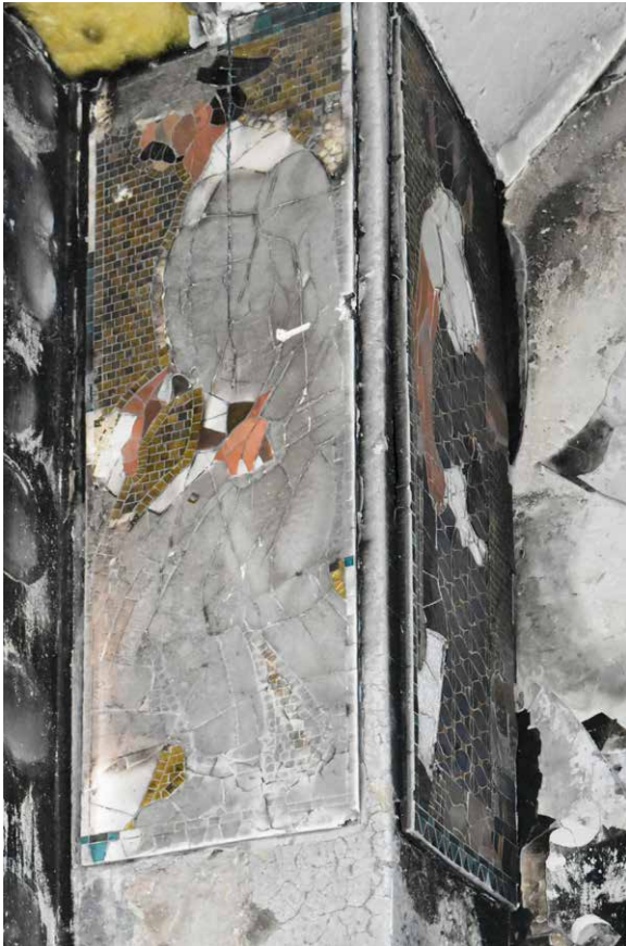
Fig. 1. Two mosaic panels after the fire, 2019. (Photo: B. Víková)
