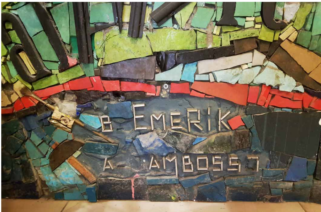
Fig. 2. Mosaic by E. Bernard and A. Tambosso in the Petrol building in Ljubljana with some pieces falling off; detail view. (Photo: B. Šeme)
