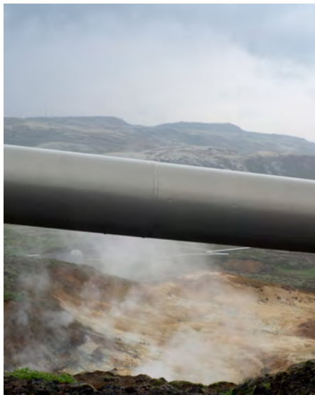
Fig. 1: Untitled, pipeline near the Nesjavallavirkjun geothermal power plant, digital photograph, 2024
